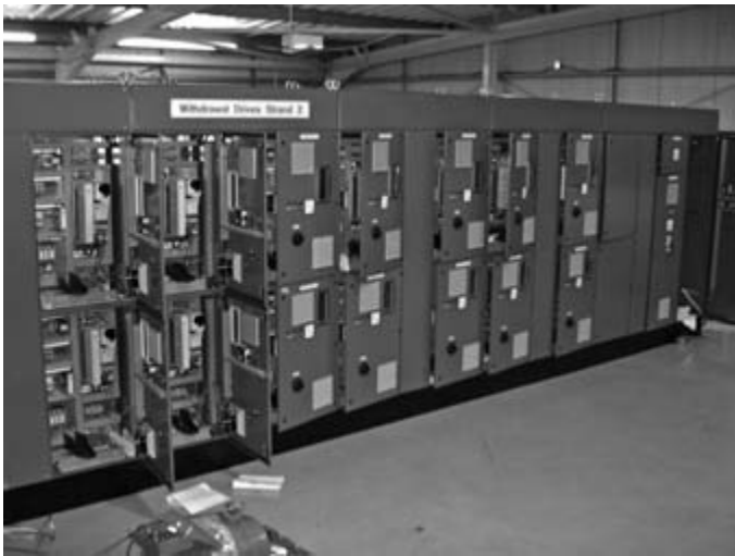
Figure C6.33 View of the roller drive control panel
