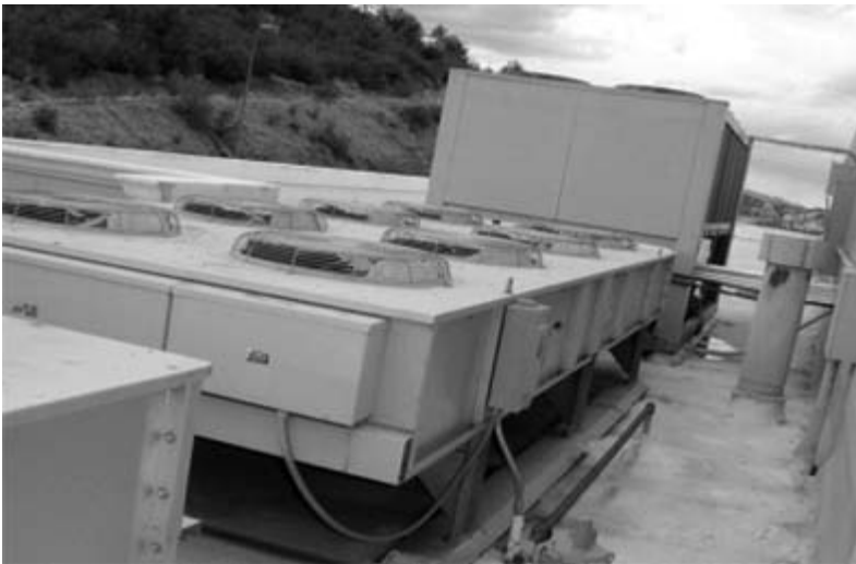
Figure C6.16 Multiple fan condenser unit
